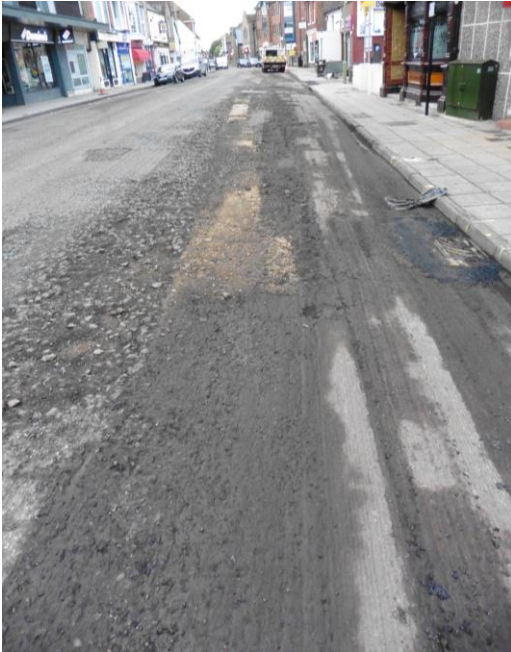
Resurfacing work in North Street in October 2016 clearly showed the route of one of the culverts running down the western side of North Street from Prince George Street to Elm Lane. Originally the Lavant Stream flowed in the open with bridges across it.
