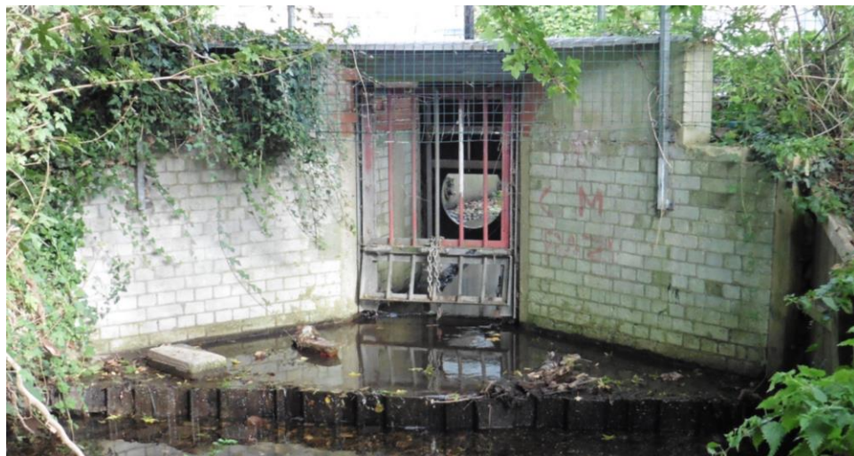
The structure at Crossland Drive housing the entrance to the pipe which diverts a large amount of the Lavant Stream to the Hermitage Stream at Stockheath Lane. Author
