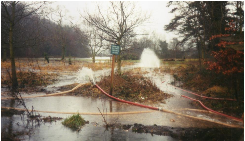
In the Sling water was coming through here at field level as well as in the ditch. It was also being pumped into there by the fire brigade.
