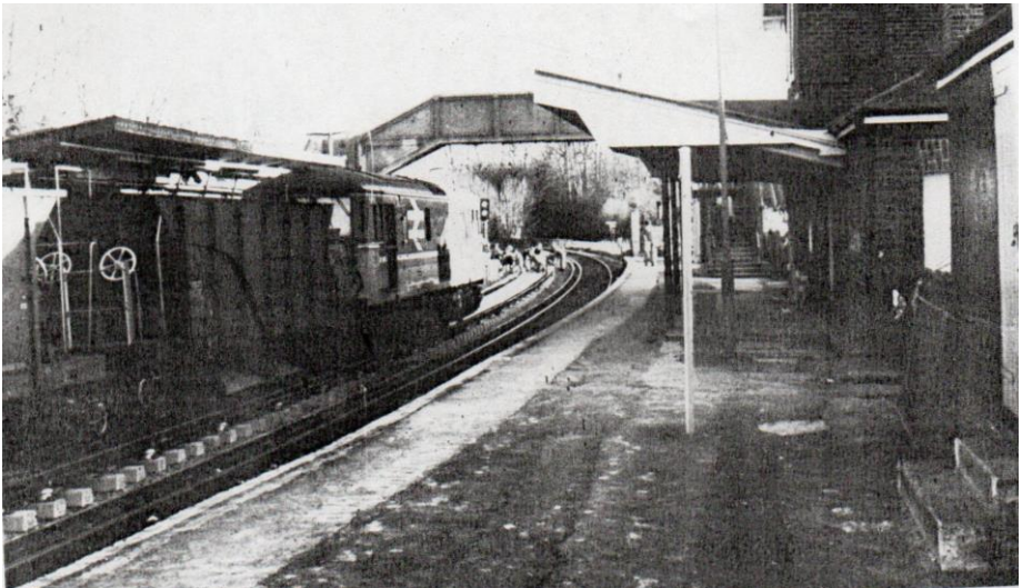
The new track and concrete sleepers have been laid and Class 73 electro-diesel locomotive heads a train consisting of giant 40 ton hopper wagons which is slowly passing over it releasing new ballast brought direct from the railway's own Meldon Quarry near Okehampton in Devon.
