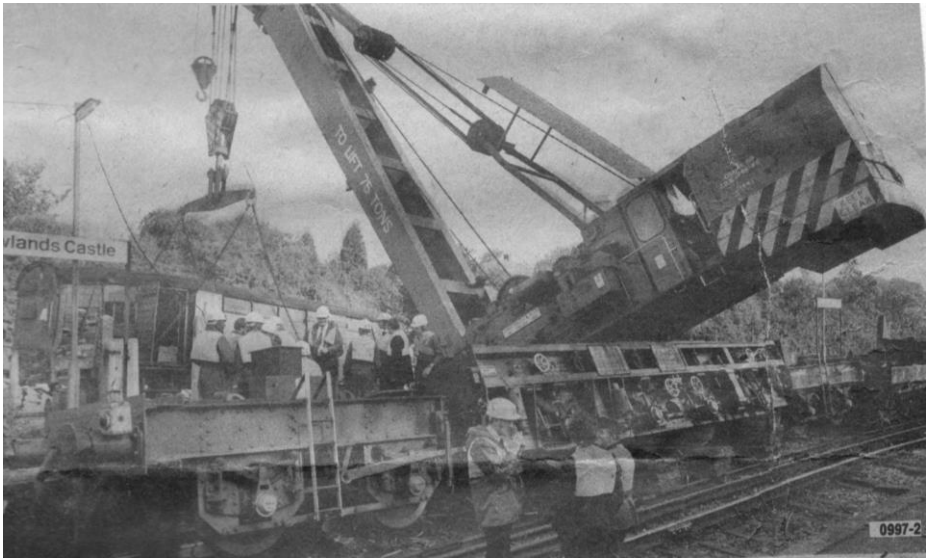
The toppled crane leaning on the Up platform
