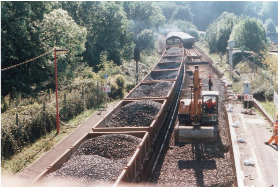
October 1995. Ballast being laid for the new Up side track. Paul Marshman
